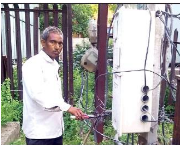
AVENGER: Srinivas cuts off the power supply to Linepar police station after he was fined Rs 500 for not wearing a helmet. Srinivas said the station, which has not paid power bills since 2016, has dues of Rs 7 lakh and this was also a violation.
